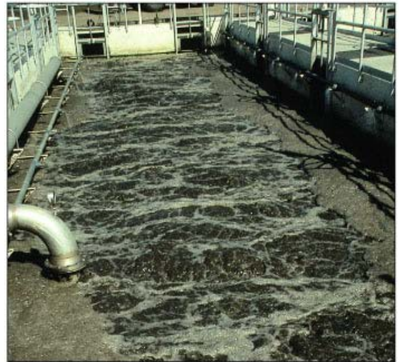
(b) An aeration tank. Note surface is frothing from aeration.
